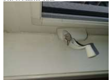
Pic. 8: Window crank handle broken
