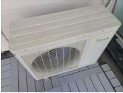
Pic. 4: AC unit
