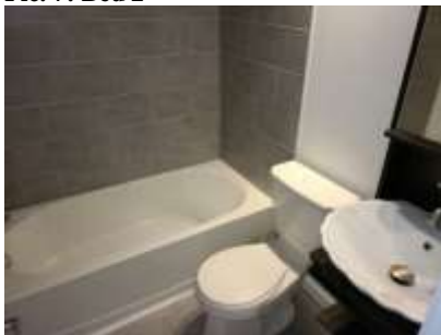
Pic. 9: 2 nd floor bath
