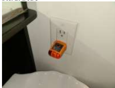
Pic. 10: Outlet doesn't trip GFCI – wired incorrectly
