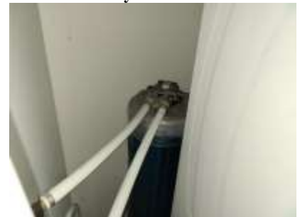
Pic. 23: Water softener
