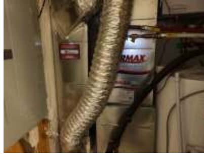
Pic. 16: Hot water furnace
