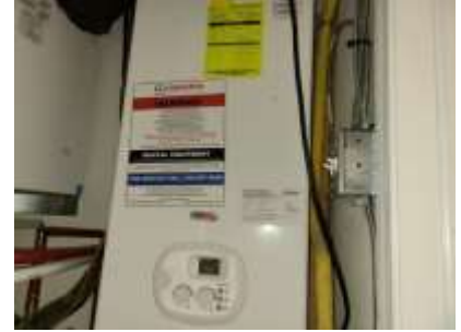
Pic. 17: Tankless boiler system
