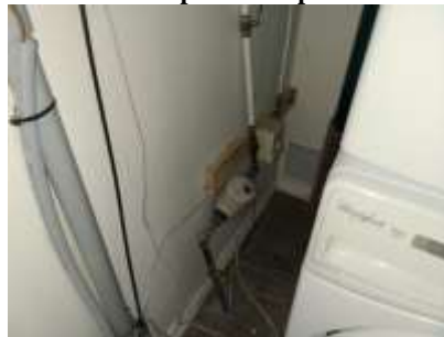
Pic. 22: Water main
