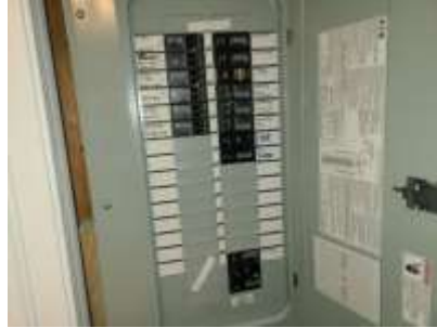
Pic. 19: 100 amp breaker panel
